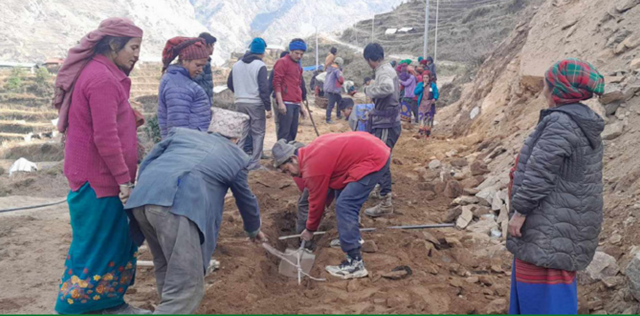
Community-led Drinking Water and Irrigation Scheme Construction in Ruby Valley, Dhading, with support from the LANN+ Project. Photo: LI-BIRD Photo Bank
